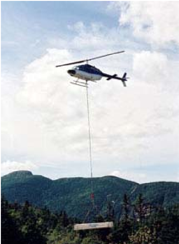
Tough site? Foard Panels being helicoptered to the top of Smugglers Notch Ski Area
